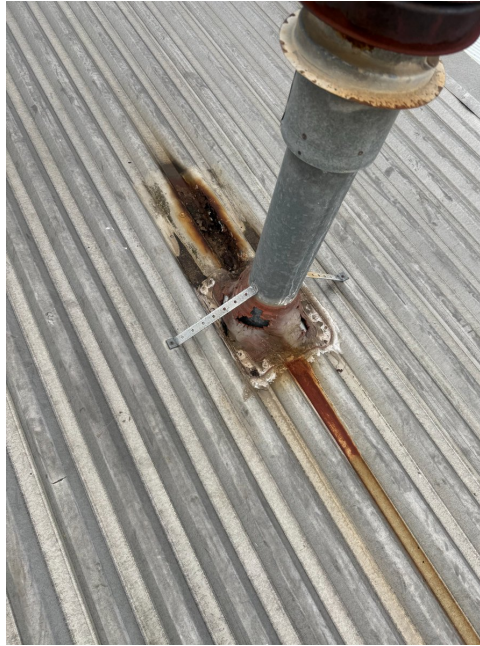
Photo: Severely corroded penetration collar with failed sealant and active rust run-off (inspection media folder 2).
