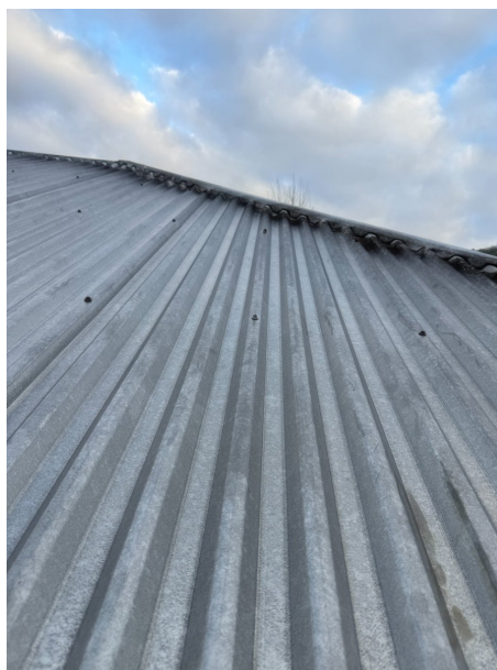
Photo: Ridge and sheet fixings – sparse and corroded (inspection media folder 4).
