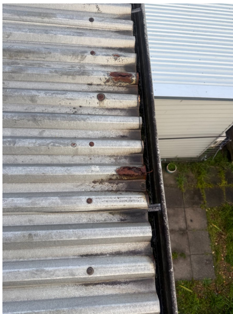
Photo: Typical roof sheet condition – missing/rusted fasteners and surface corrosion (inspection media folder 1).
