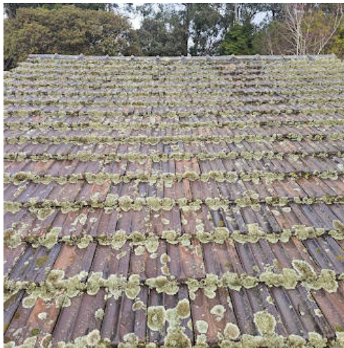
Picture 3: Different angle of roof that shows how dirty the roof is with moss growing on it that will require high pressure cleaning.
