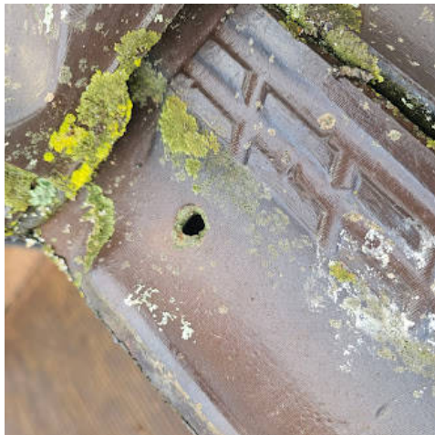
Picture 7: Showing existing poor conditions of some tiles with holes in it that will require to be sealed and water tight.
