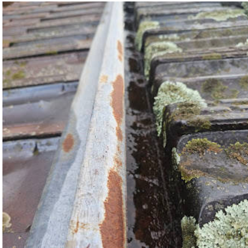
Picture 9: Showing gutters and flashings in poor condition that will require to be changed due to rust and water leaks.
