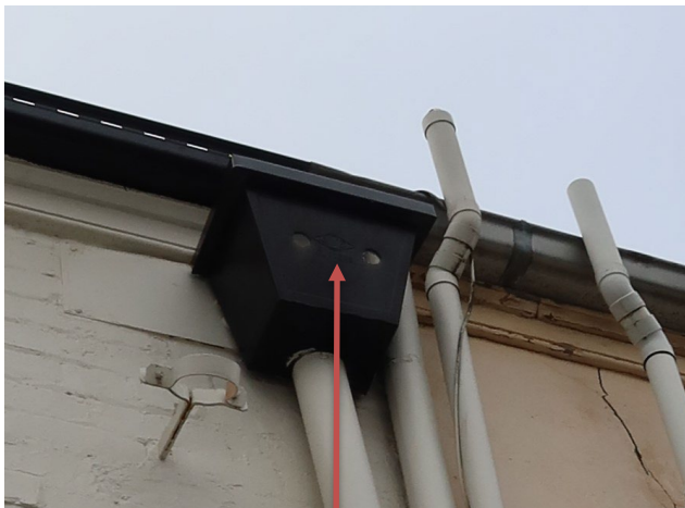
9. The rainhead overflows are undersized and too high.
