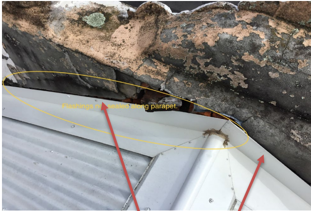
2. (RN Plumb. Photo) The apron flashing has not been installed correctly.
