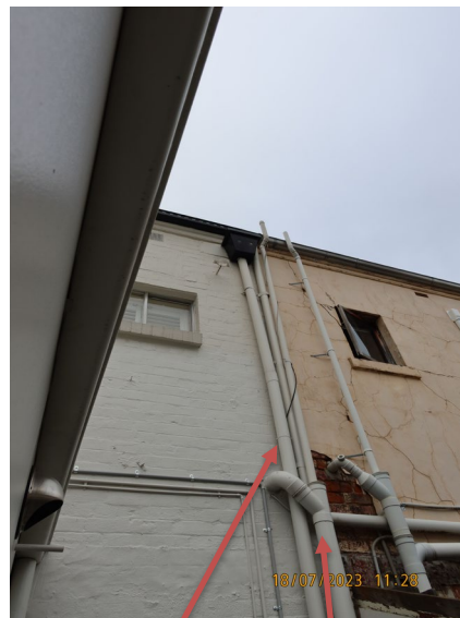
10. The downpipes are required to be supported at maximum 2000mm spacings. This applies to all the relevant downpipes etc.
