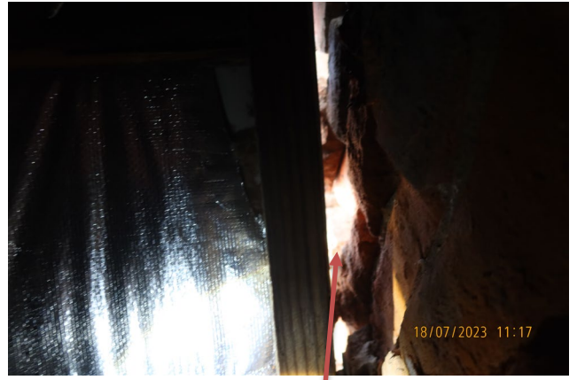
3. The apron parapet flashing has not been installed correctly.
