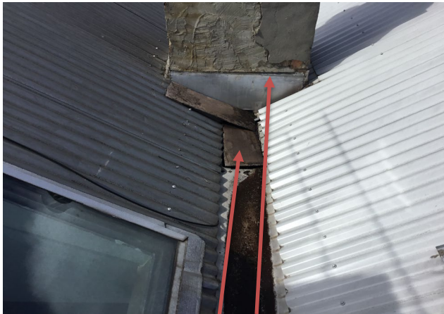
8. (PN Plumb photo) The chimney has not been flashed correctly, note rubbish that has been left in the boxgutter.
